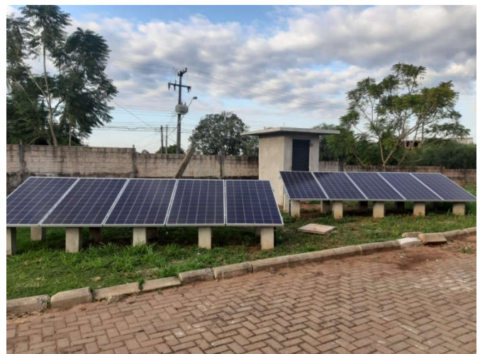
Figure 1. Photovoltaic system installed at Unioeste
