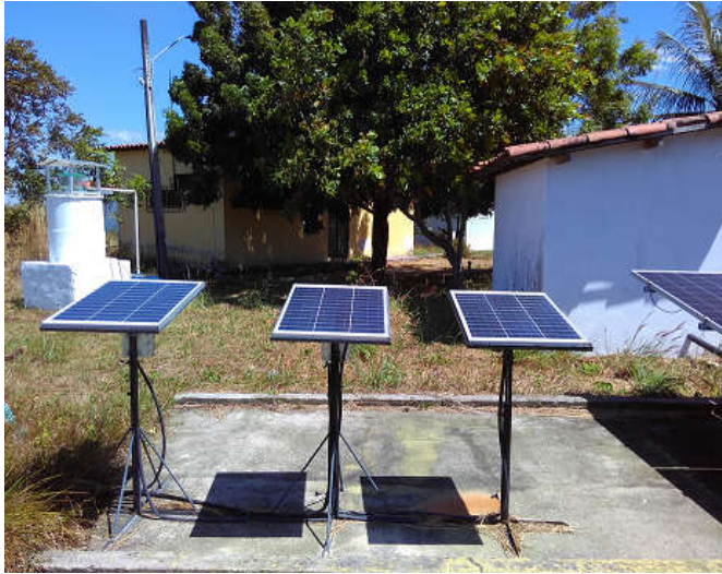
Fig. 1. Picture of three photovoltaic modules installed
