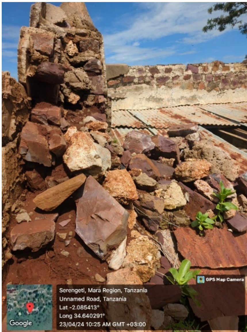
Figure 5. The picture showed a collapsed stone masonry wall
