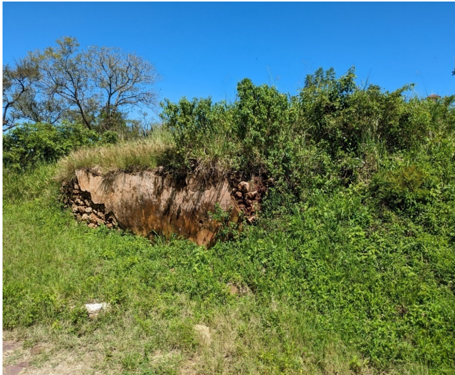
Figure 4. The picture shows the foundation wall that was built by sample 2A
